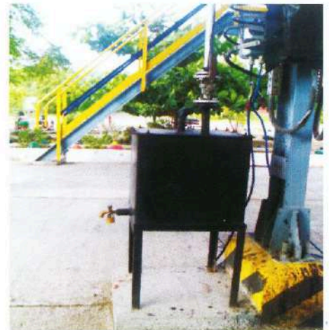
Funnel arrangement with collection box provided to check spillage at Tank Lorry Filling Gantry in Manmad Installation
